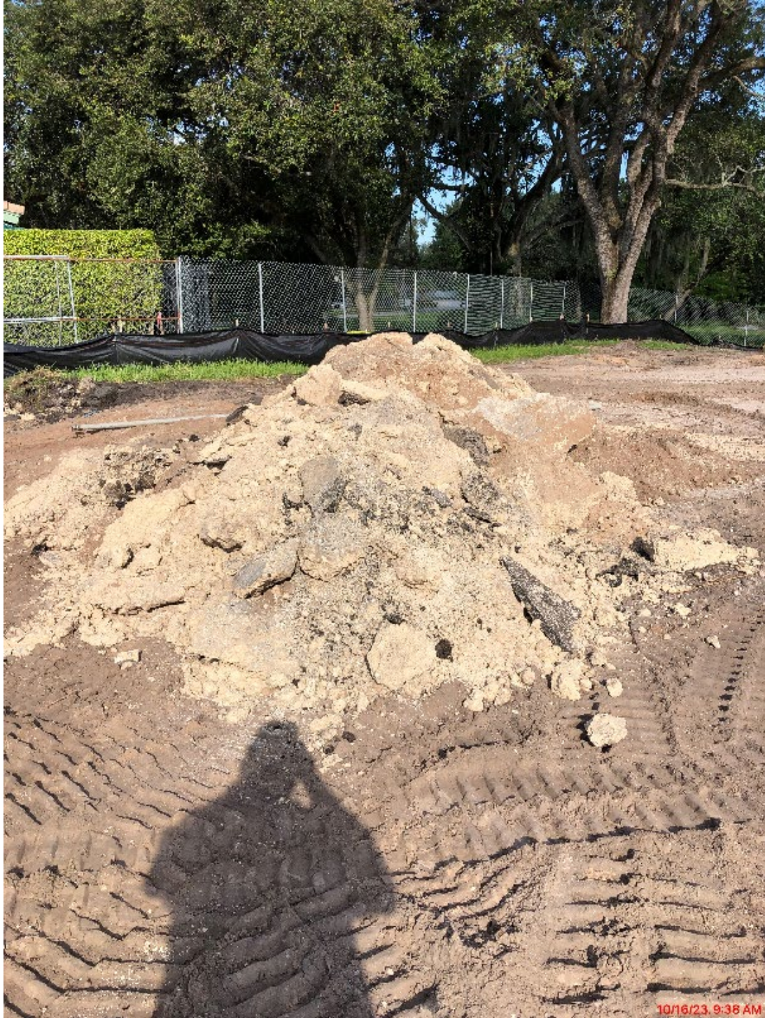
Concrete and Asphalt walks and debris
