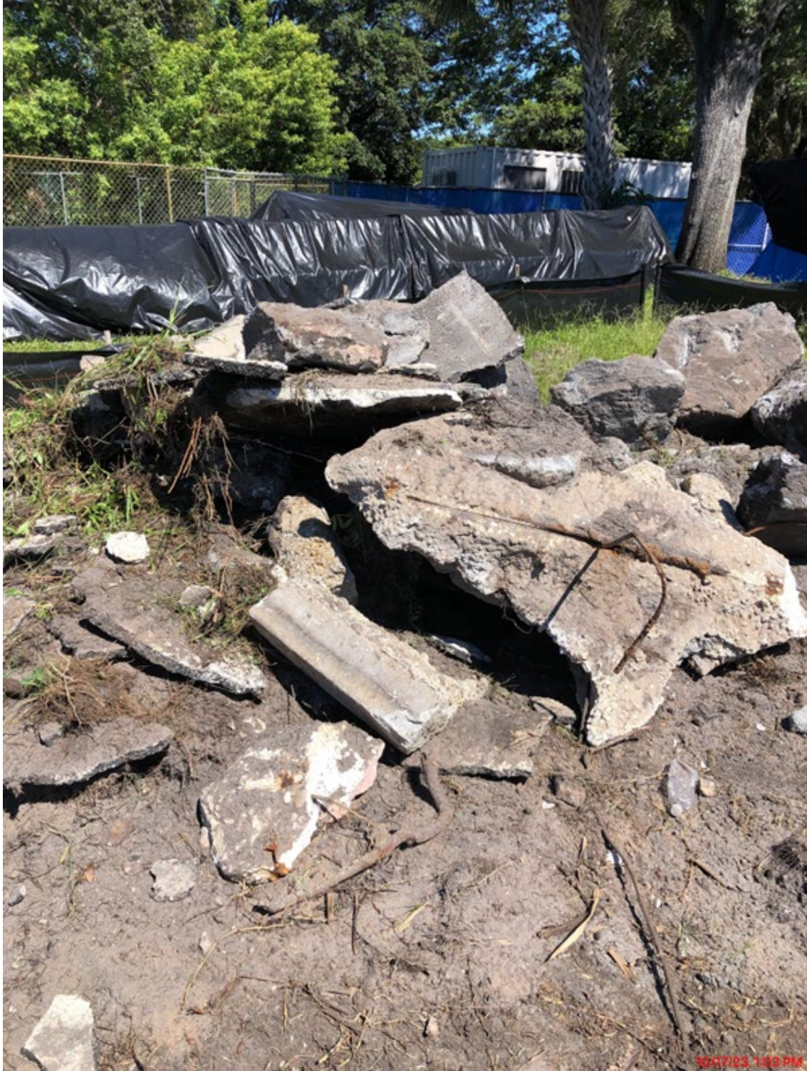
Concrete and Asphalt walks and debris
