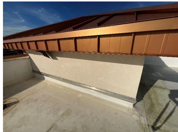
Photo 41 – Main Roof – Tower Walls Overall view of the metal Tower Roof eave fascia condition.
