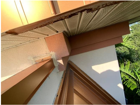
Photo 31 – Main Roof – Tower Walls Overall view of Corner Tower decorative foam trim band.
