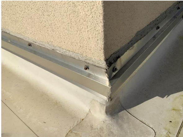
Photo 13 – Main Roof – Interior Tower Walls Overall view of the existing conventional stucco counter-flashing condition.
