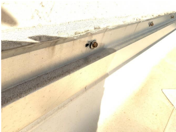
Photo 14 – Main Roof – Interior Tower Walls Overall view of the existing TPO roof counter-flashing condition.
