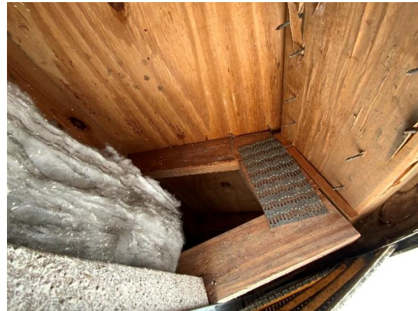
Photo 35 – Main Roof – Tower Walls Overall view of the soffit condition.
