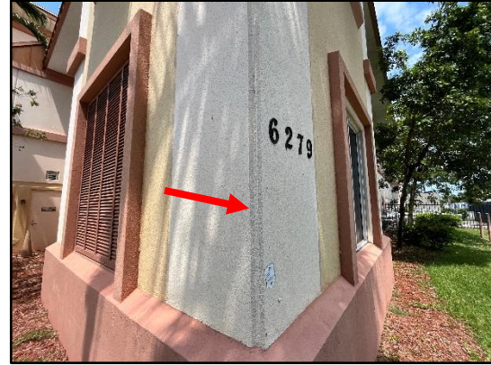
Figure 17 – Overall view of an outside corner panel wall joint to be removed and replaced.
