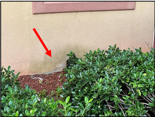
Figure 13 – Overall view of the existing exterior coating condition along the tilt-up panel walls.
