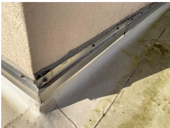
Photo 51 – Main Roof – Tower Walls Overall view of the metal roof counterflashing needing sealant at the TPO interface.
