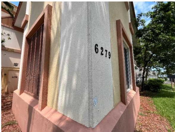
Photo 56 – Exterior Tilt-Up Walls Overall view of an outside corner panel wall joint to be removed and replaced.
