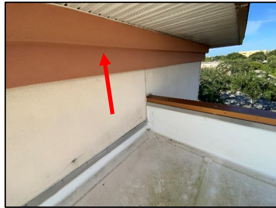
Figure 9 – Overall view of the existing foam trim bands along the Center West Tower.
