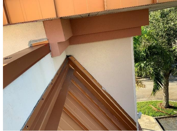
Photo 28 – Main Roof – Tower Walls Overall view of Corner Tower decorative foam trim band.
