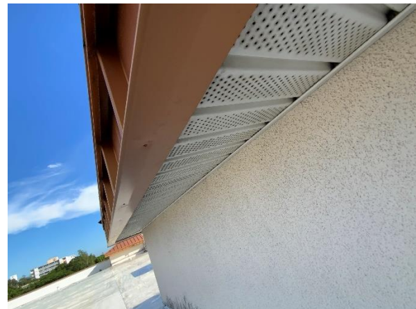
Photo 53 – Main Roof – Tower Walls Overall view of the soffit vent sealant installation interface.
