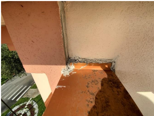
Photo 21 – Main Roof – Interior Tower Walls Overall view of the parapet coping cap to adjacent conventional stucco wall transition.
