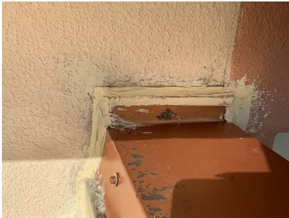
Photo 26 – Main Roof – Interior Tower Walls Overall view of the parapet coping cap to adjacent conventional stucco wall transition.
