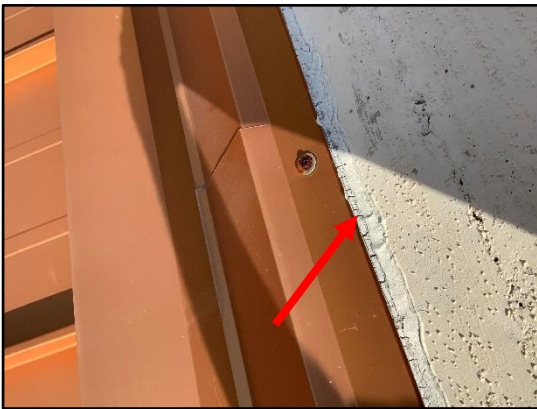
Figure 14 – Overall view of sealant to be replaced at metal roof headwall flashing.
