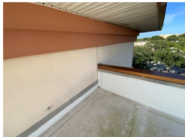
Photo 30 – Main Roof – Tower Walls Overall view of West Center Tower decorative foam trim band.
