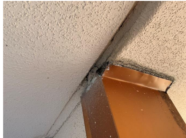
Photo 23 – Main Roof – Interior Tower Walls Overall view of the parapet coping cap to adjacent tilt-up wall transition.
