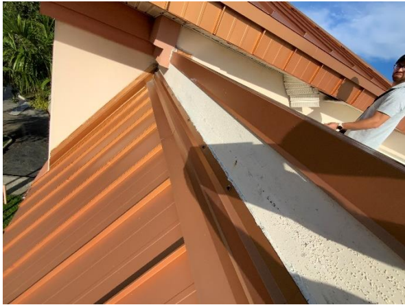
Photo 43 – Main Roof – Parapet Walls Overall view of the exterior parapet wall to be recoated.
