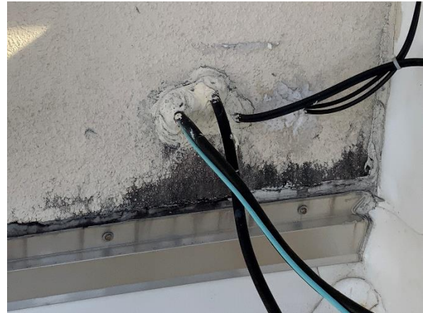
Photo 16 – Main Roof – Interior Tower Walls Overall view of the wire penetrations in the conventional stucco system.
