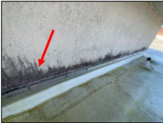
Figure 12 – Overall view of the existing exterior coating condition along the conventional stucco.
