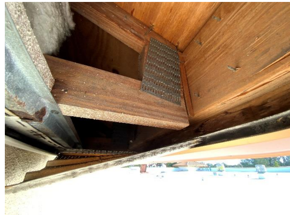
Photo 36 – Main Roof – Tower Walls Overall view of the soffit condition.
