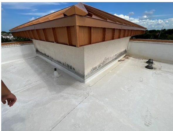
Photo 45 – Main Roof – Tower Walls Overall view of the exterior framed Tower walls to be recoated.
