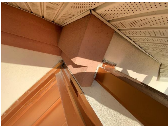
Photo 27 – Main Roof – Tower Walls Overall view of Corner Tower decorative foam trim band.
