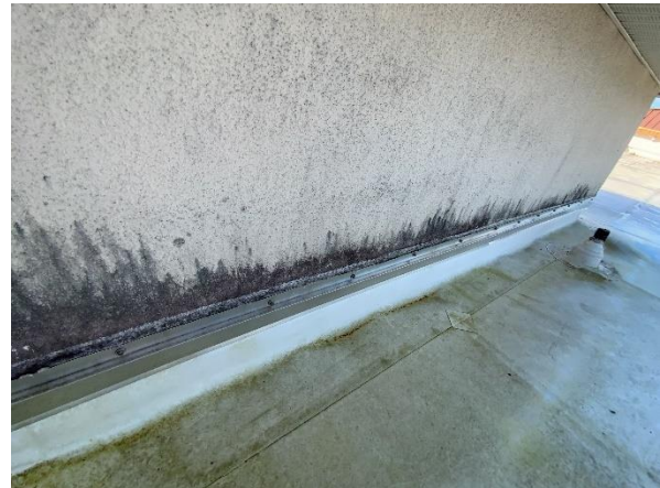
Photo 17 – Main Roof – Interior Tower Walls Overall view of the existing conventional stucco counter-flashing condition.
