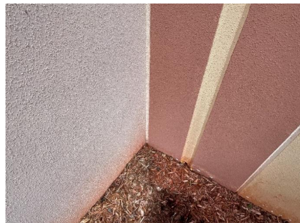
Photo 54 – Exterior Tilt-Up Walls Overall view of an inside corner panel wall joint to be removed and replaced.
