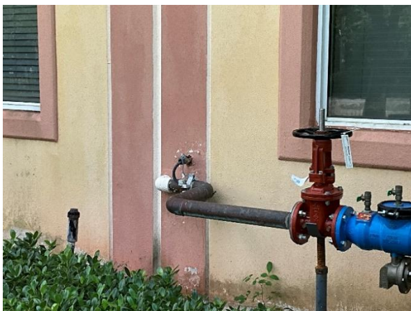
Photo 57 – Exterior Tilt-Up Walls Overall view of a vertical panel wall joint to be removed and replaced.
