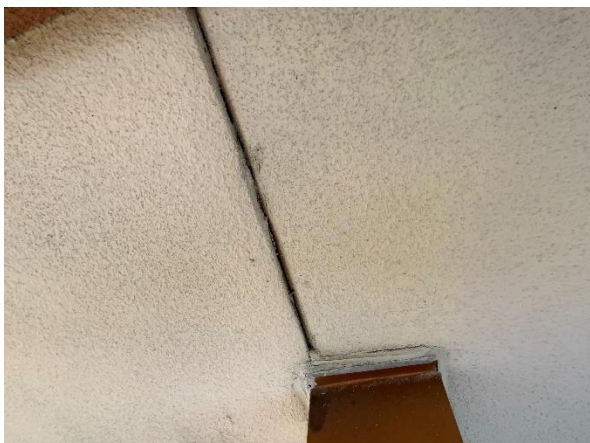
Photo 15 – Main Roof – Interior Tower Walls Overall view of the existing conventional stucco to tilt-up wall transition.
