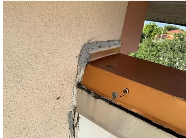
Photo 22 – Main Roof – Interior Tower Walls Overall view of the parapet coping cap to adjacent conventional stucco wall transition.
