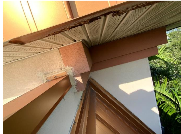
Photo 40 – Main Roof – Tower Walls Overall view of the damaged metal Tower Roof eave fascia condition.
