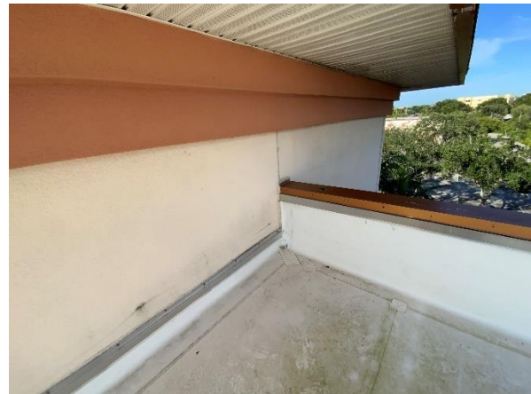
Photo 24 – Main Roof – Interior Tower Walls Overall view of the parapet coping cap to adjacent tilt-up wall transition.
