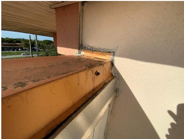
Photo 20 – Main Roof – Interior Tower Walls Overall view of the parapet coping cap to adjacent conventional stucco wall transition.
