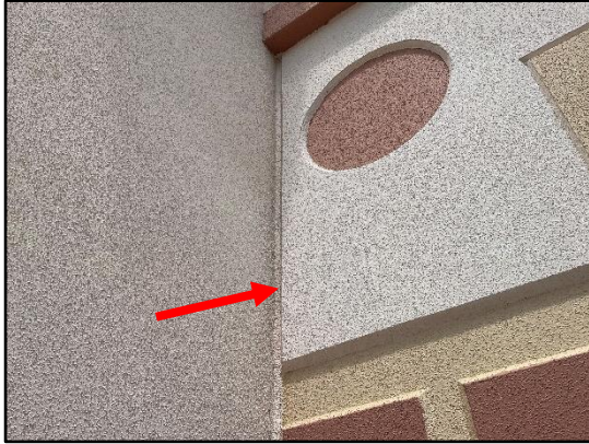
Figure 16 – Overall view of an inside corner panel wall joint to be removed and replaced.
