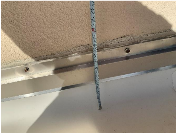
Photo 19 – Main Roof – Interior Tower Walls Overall view of the existing TPO roof counter-flashing measurements.
