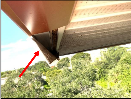
Figure 11 – Overall view of damaged roof fascia.
