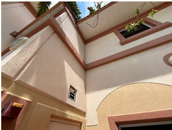
Photo 44 – Exterior Tilt-Up Walls Overall view of the exterior tilt up walls to be recoated.
