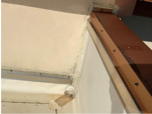
Photo 25 – Main Roof – Interior Tower Walls Overall view of the parapet coping cap to adjacent conventional stucco wall transition.
