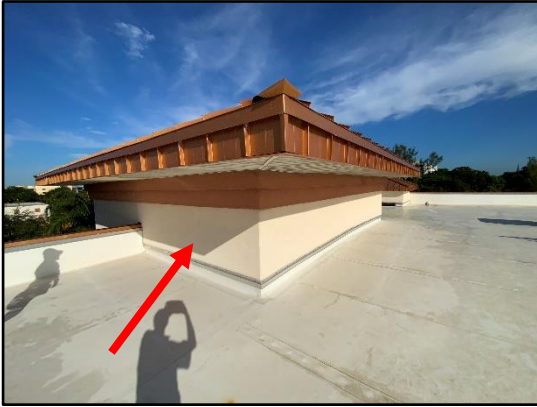
Figure 4 – Overall view of the conventional stucco on the Roof Tower interior walls.
