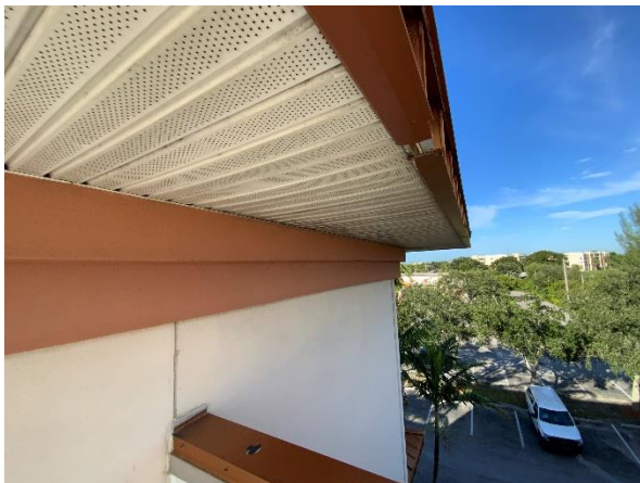
Photo 38 – Main Roof – Tower Walls Overall view of the damaged metal Tower Roof eave fascia condition.
