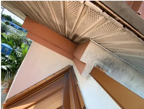
Photo 32 – Main Roof – Tower Walls Overall view of Corner Tower decorative foam trim band.
