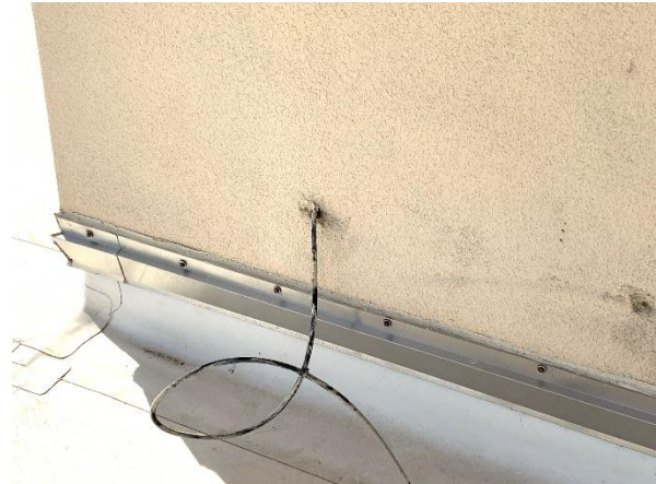
Photo 52 – Main Roof – Tower Walls Overall view of the wire penetrations sealant installation.
