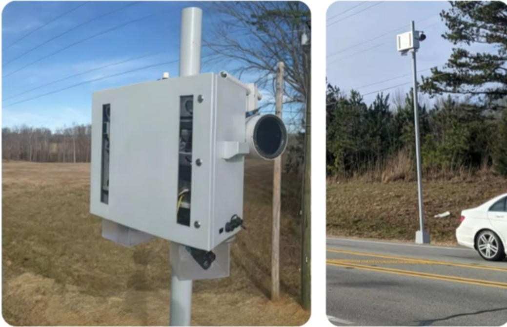
Figure 19: Installed Speed - LiDAR System
