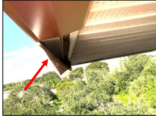
Figure 11 – Overall view of damaged roof fascia.
